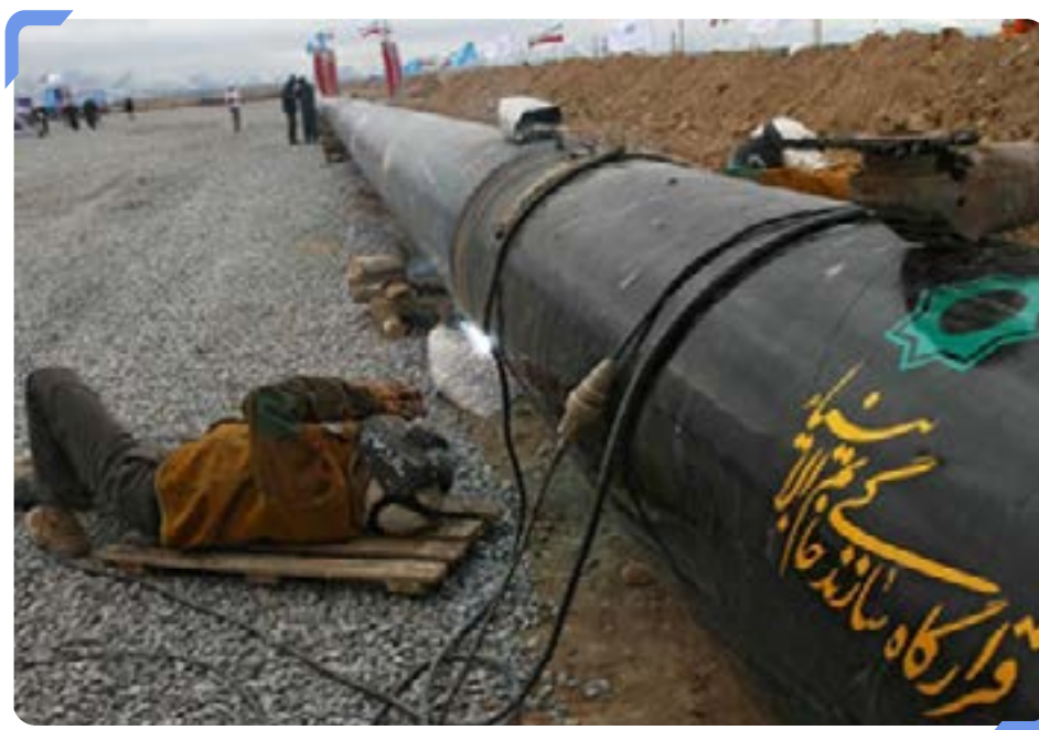
Khatam al-Anbiya Construction Headquarters is one of the largest contractors in upstream and downstream projects in the oil, gas, and petrochemical industries.
